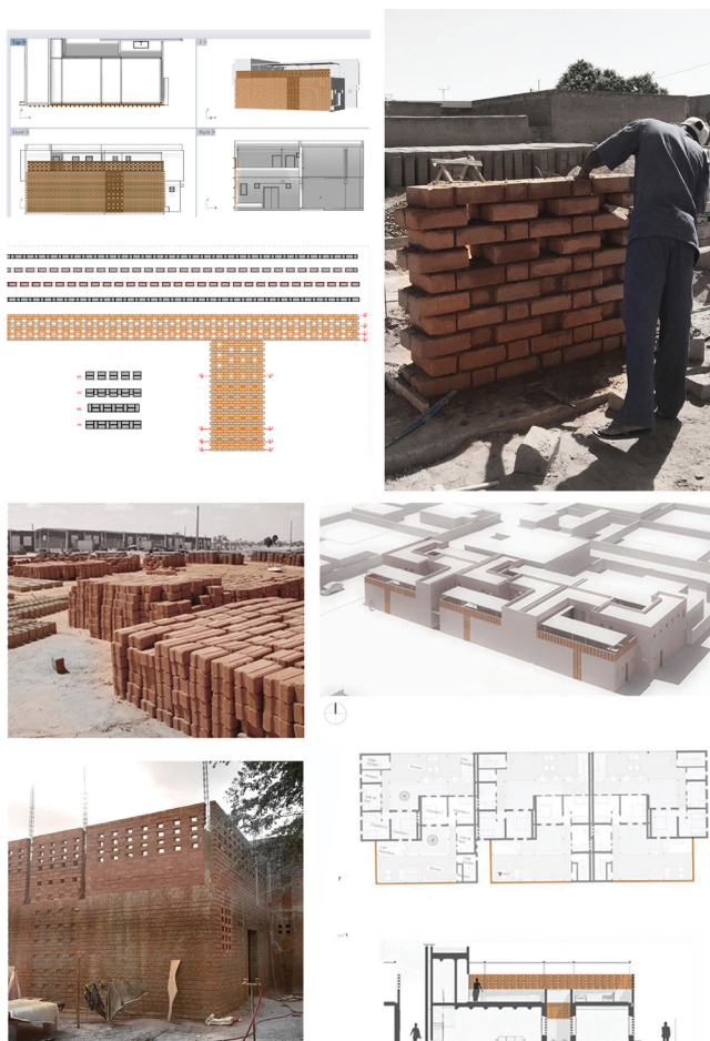
Figure 4, the process of digital design, and construction of the brick screens in Niamey, Niger. Image credit: united4design
